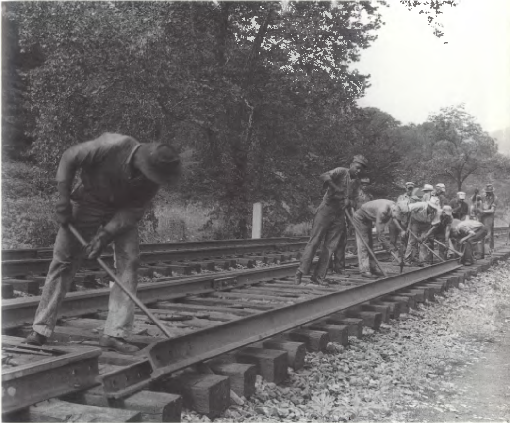
A railroad gang kicks out a length of rail near Thayer, West Virginia, 1944 (Courtesy Chesapeake & Ohio Railway)
